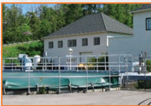
Wastewater Treatment Plant • La Malbaie
