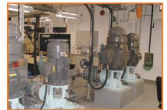
Tank and booster post • Paspébiac
