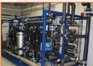
Potable water treatment • Lac Bouchette et Ermitage St-Antoine
